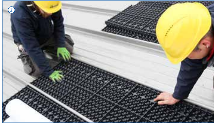
Put the Urbanscape drainage and storage layer onto RIB-ROOF profiled sheets. Make sure that the edges are put under the sheet seams.
