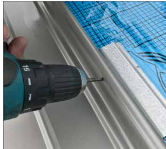
2. Drill a lateral hole on the circular seam at an angle of approx. 45°
