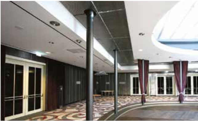
Chilled ceiling, Hotel Steigenberger Drei Mohren, Augsburg, Germany. Architect: Alpstein. Mesh: Atlantic (5)
